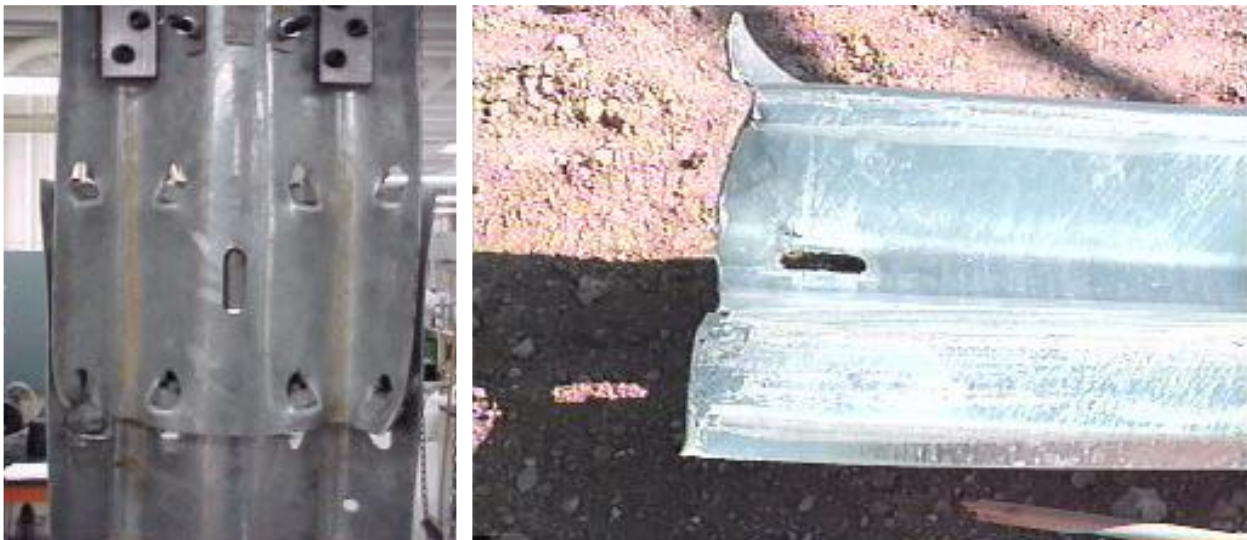
Figure 84. Rail Splice Failures: Quasi Static Tensile Test Results (Left) and TTI Full-Scale Testing Results (Right) [74,75]
