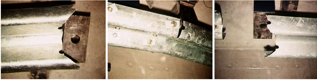
Figure 86. Rail Rupture from Quasi-Static Tension Testing at MwRSF [77]
