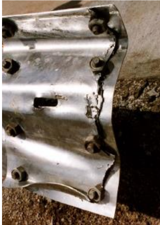
Figure 85. Ruptured Rail Installed Over a Curb [76]
